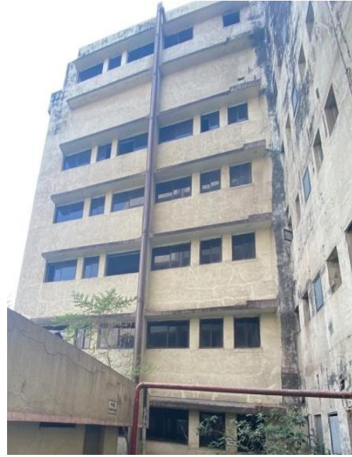
Face F: minor surface cracks on plaster & black moss formation has been observed on wall at all floors.
