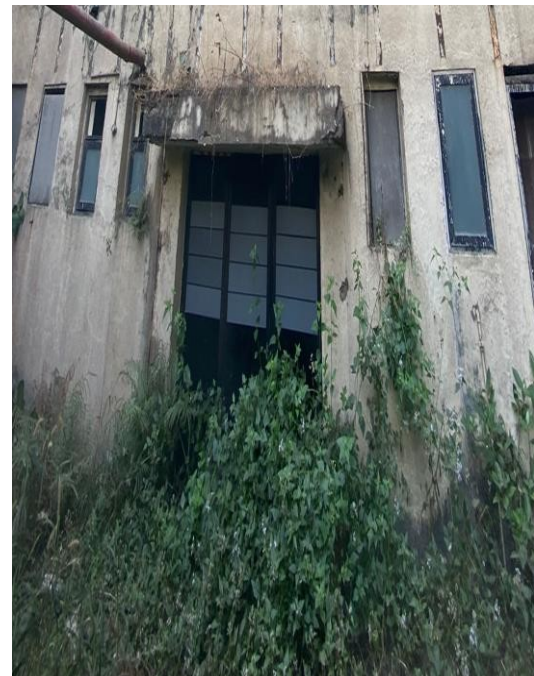
Face E: Vegetation growth has been observed on plinth protection at ground floor.
