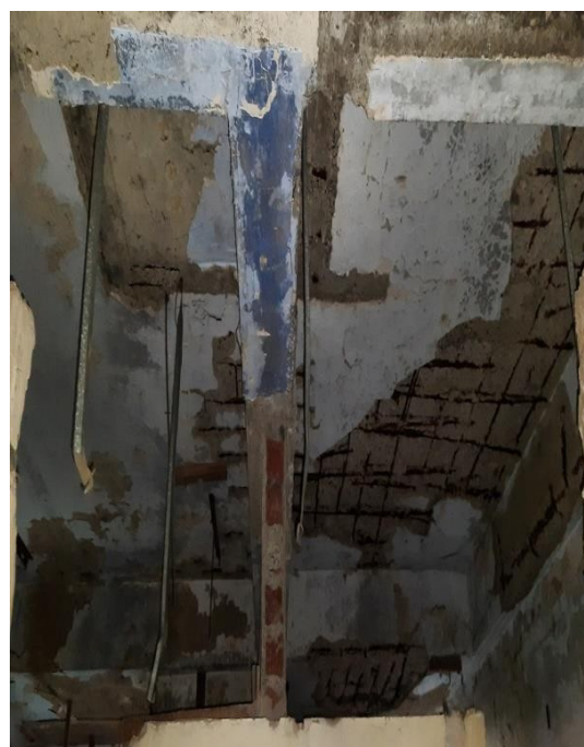
Spilling of cover concrete & exposed corroded & broken reinforcement has been observed on slab.
