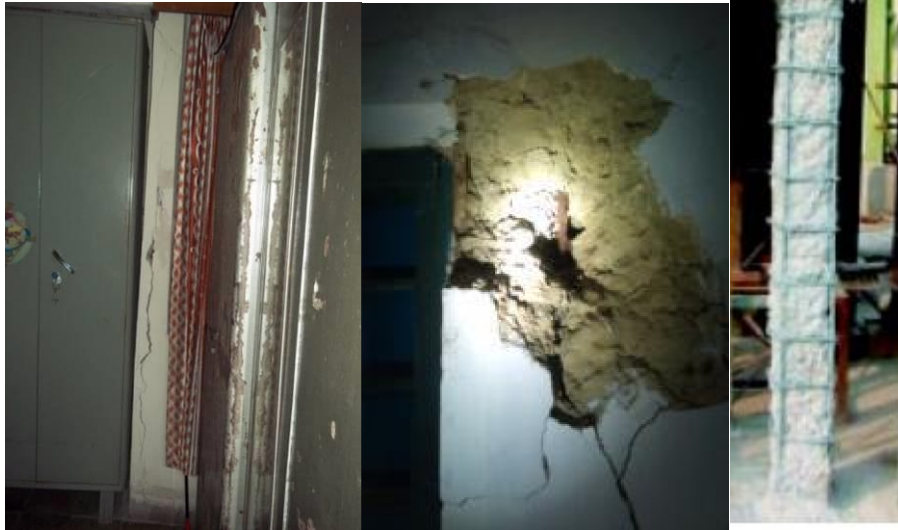
Fig.1. Damaged column a) and b) Before removal of cover concrete and c) After removal of cover concrete
