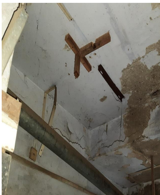
Corrosion crack and air pocket has been observed on Beam.
