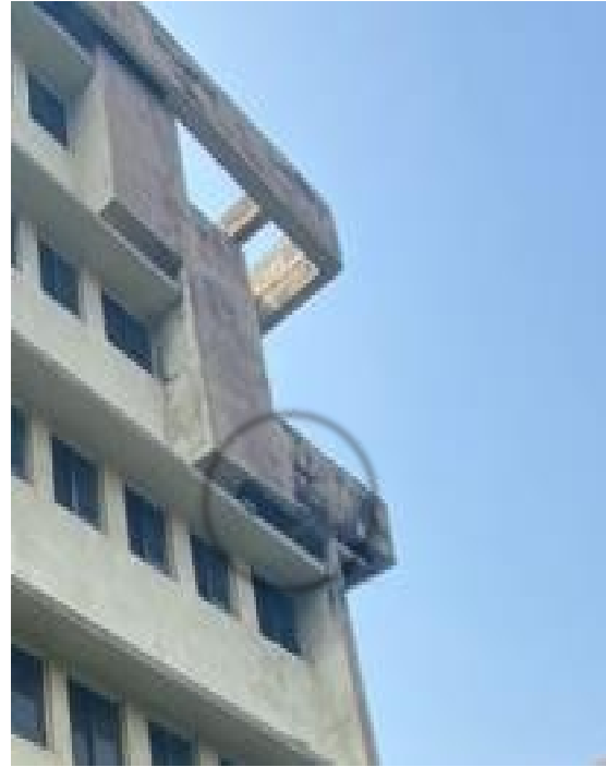
Face C: Spilling cover concrete & exposed reinforcement has been observed at 4th floor balcony slab.
