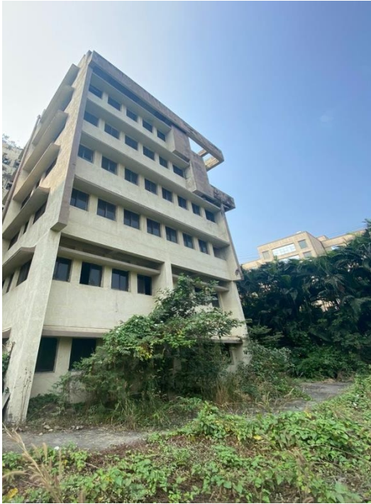
Face C: Full view, surface cracks on plaster has been observed on wall at all floors. & vegetation growth has been observed on plinth protection.
