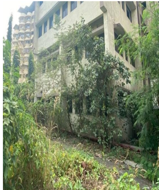
Face G: Vegetation growth has been observed on plinth protection at ground floor.
