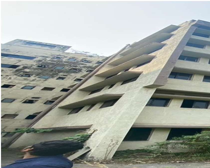
Face D: Full view, minor plaster surface cracks has been observed at few locations.
