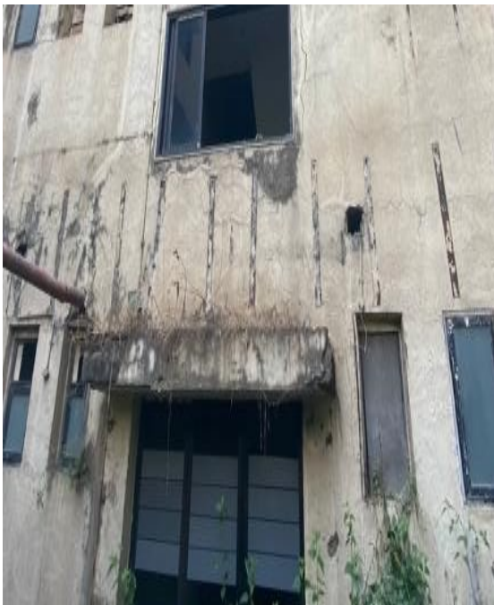
Face E: Spilling cover concrete & exposed reinforcement has been observed at ground floor Chajja.
