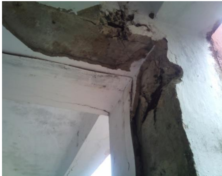
Fig: 7 Damaged Beam
