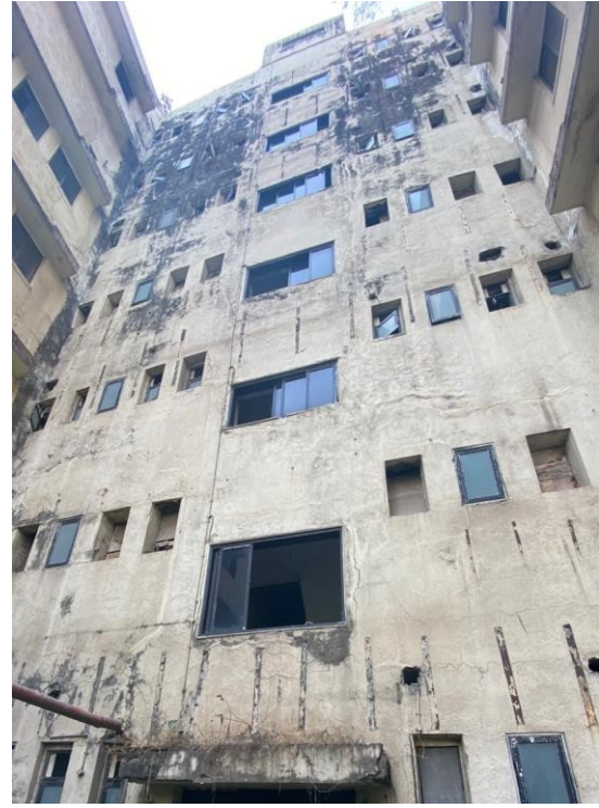
Face E: Surface cracks on plaster & black moss formation has been observed on wall at all floors.
